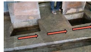
Fig. 2. Silt trap tanks
